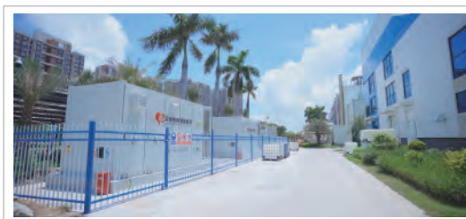
Zhuhai Great Power Production 29.77MWh Project
