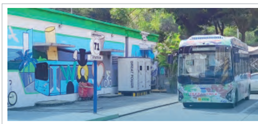
Croatia 17MWh Photovoltaic and Storage Complementary Project
