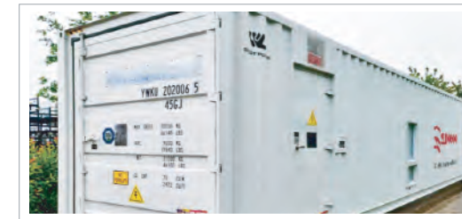
Croatia 17MWh Photovoltaic and Storage Complementary Project
