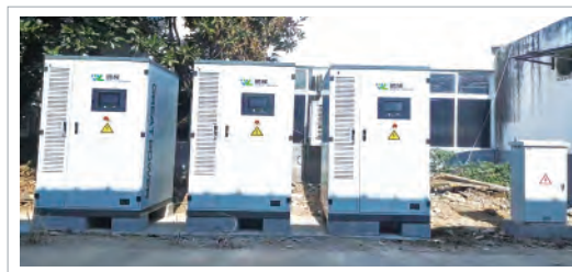
Runan Yuxin 1.5MWh Project
