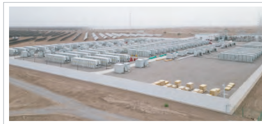
Bachu 140MWh Agro-Photovoltaic Complementary Project
