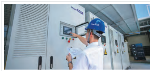
Guangzhou Xinli 2.33MWh Project
