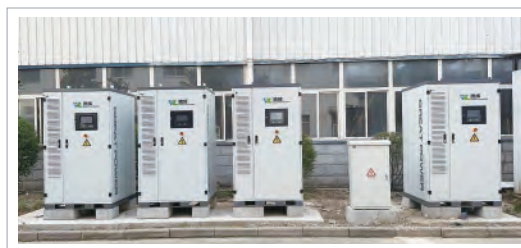
Zhumadian Zhongji Huajun 2.8MWh Project
