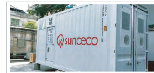
Marinska 1MWh Malin Hotel Project
