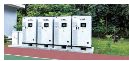
Shenzhen Yinghe 3.26MWh Project
