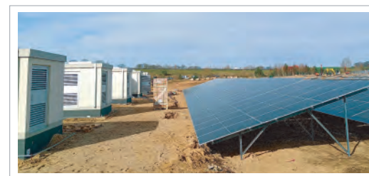
Germany 16.77MWh Containerized Energy Storage Project
