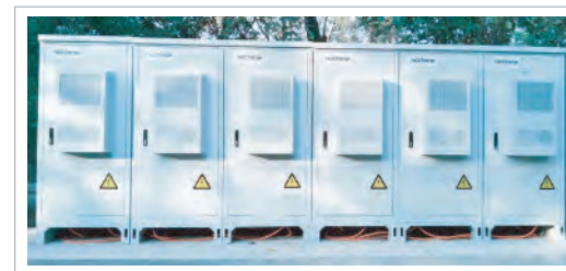
India 2MWh High-Grid Photovoltaic Storage Project
