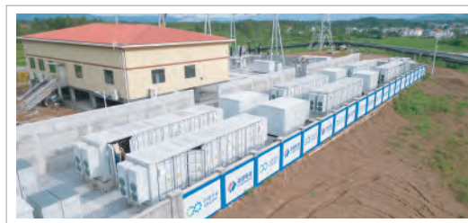
Ji'an 15MWh Agro-Photovoltaic Complementary Project
