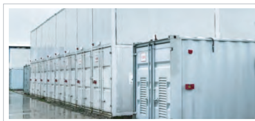
State-Owned Shipyard 100MWh Energy Storage Station Project
