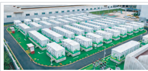
Nanning 100MWh Energy Storage Project
