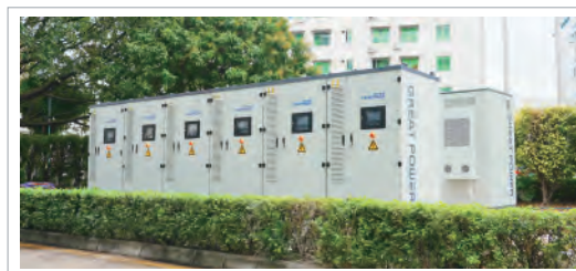
Guangzhou Production 7.33MWh Project
