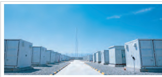
Jimusaer 150MWh Project
