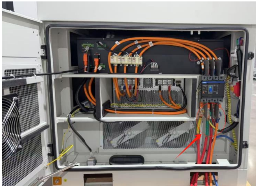
AC wiring interference
